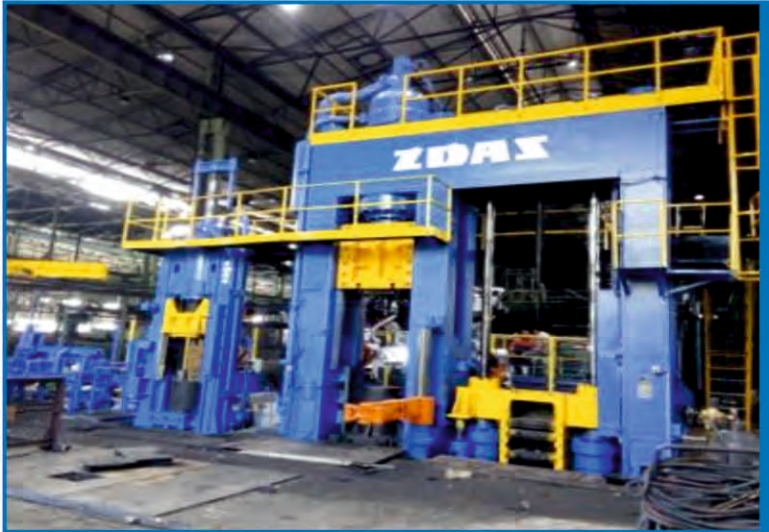
ROBOTIC FORGING PLANT CZ - II
